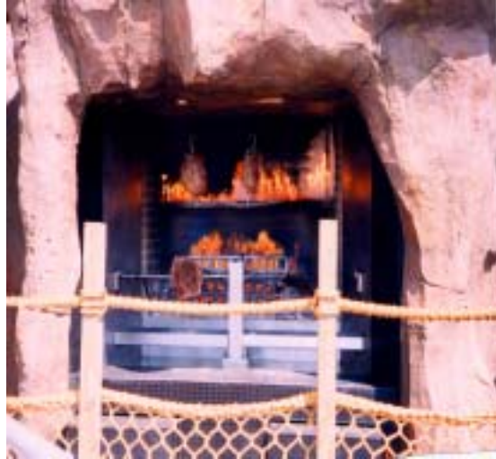
This giant rotisserie was built into a "cave" at Shipwreck Island at Sea World San Diego and features horizontal and vertical spits. It stands 12 ft. wide, 6 ft. deep, and 11 ft. high!
